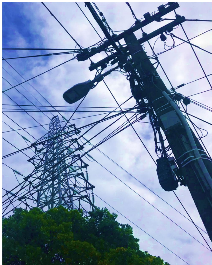
Transmission and distribution lines, Wellington, New Zealand
