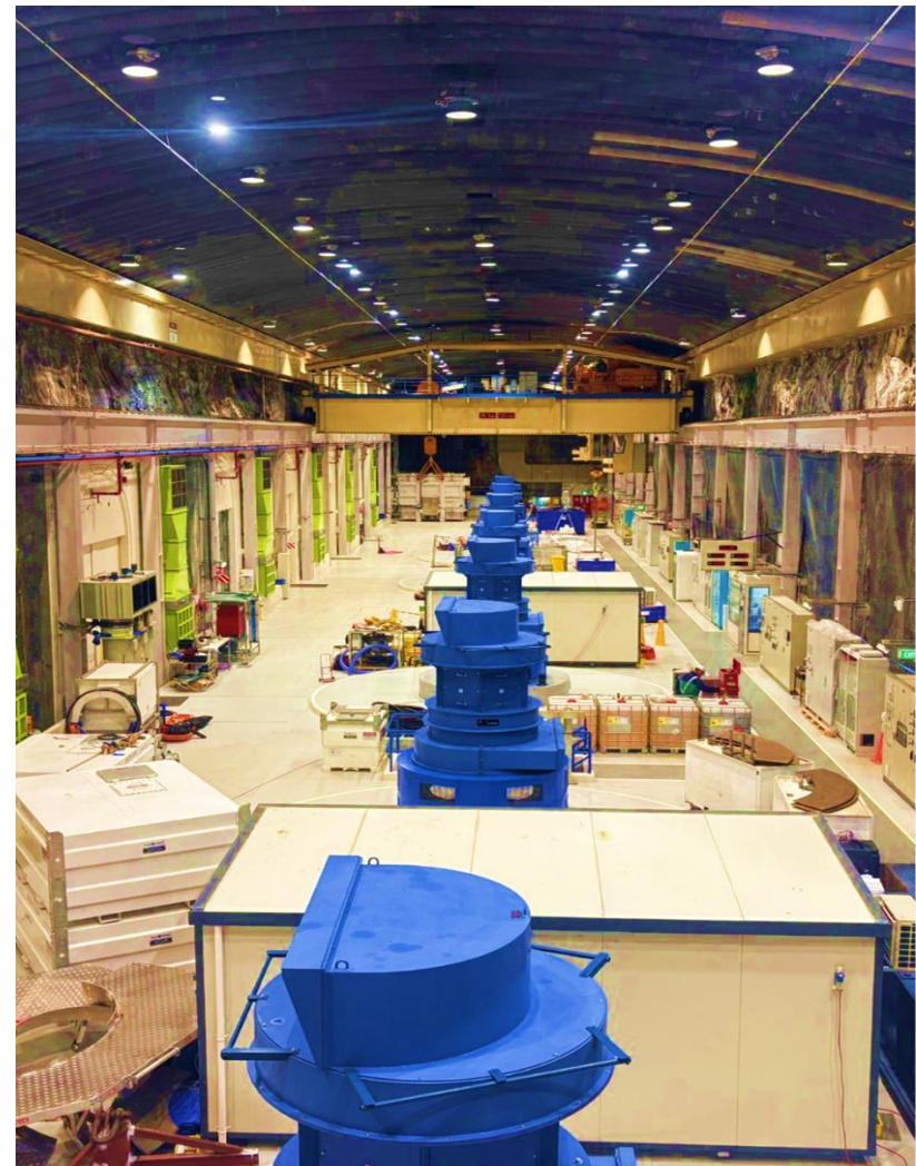
Synchronous generators - turbine hall, Manapouri power station
