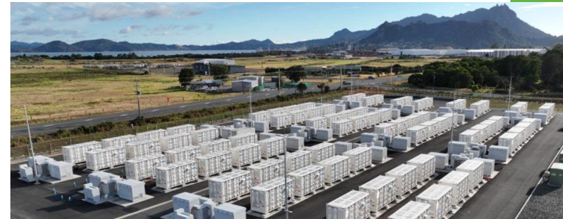
Installed BESS of 235MW / 435 MWh expected to increase to
